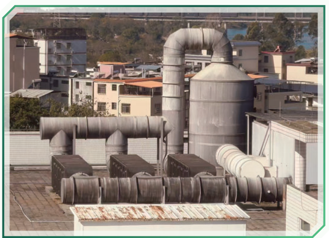
HYN2 waste gas collection and purification facilities in Heyuan plant
