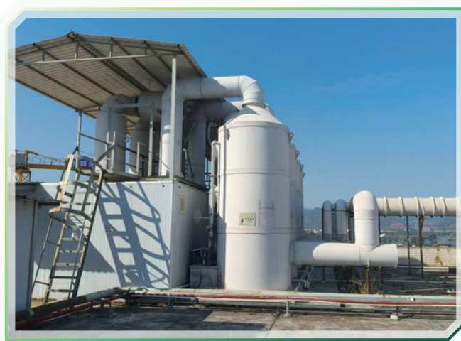
HYN1 waste gas collection and purification facilities in Heyuan plant
