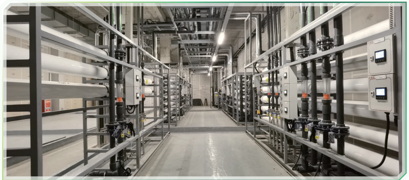
Pure water preparation system
